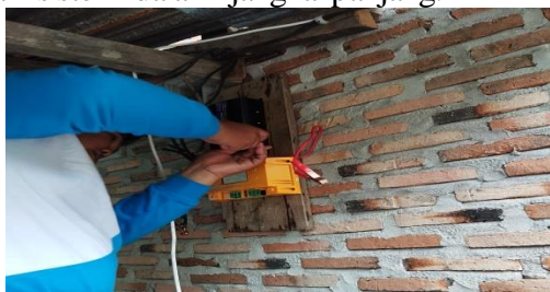
Gambar 6. Perakitan Solar Charge Controller (SCC) dan inverter
